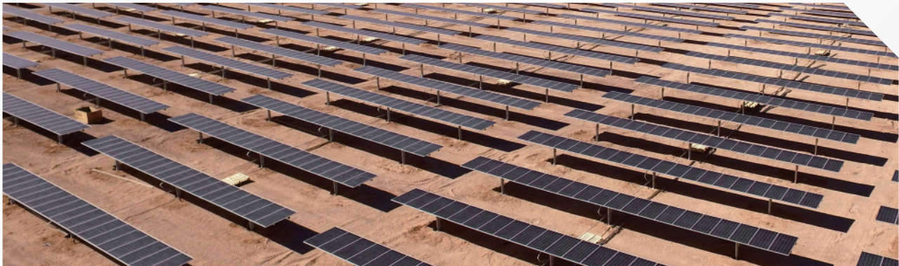
40+MW 📍 Project Location: Syria 📋 Module Type: Solar N Plus N-Type 580W 📅 On-grid Date: 2024.5
