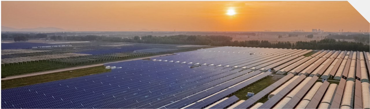
20MW 📍 Project Location: Lujiang, China 📋 Module Type: Solar N Plus N-Type 560W 📅 On-grid Date: 2023.4
