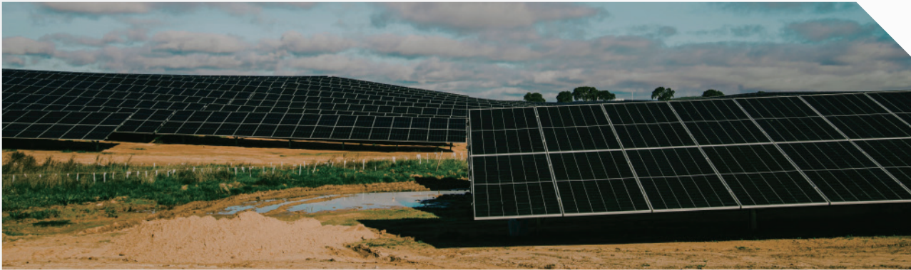
25MW 📍 Project Location: Romania 📋 Module Type: Solar N Plus N-Type 630W 📅 On-grid Date: 2025.10
