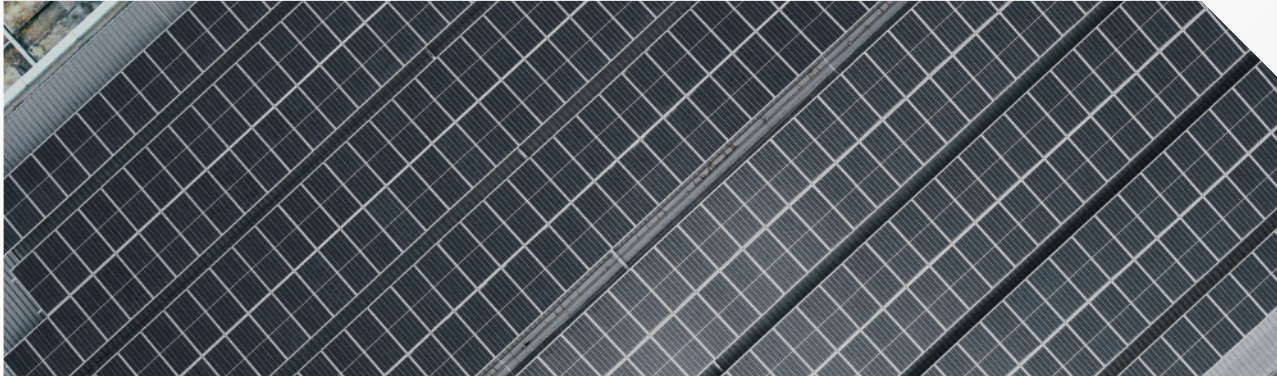
27.6MW 📍 Project Location: Suqian, China 📋 Module Type: Solar N Plus N-Type 580W 🕒 On-grid Date: 2023.2
