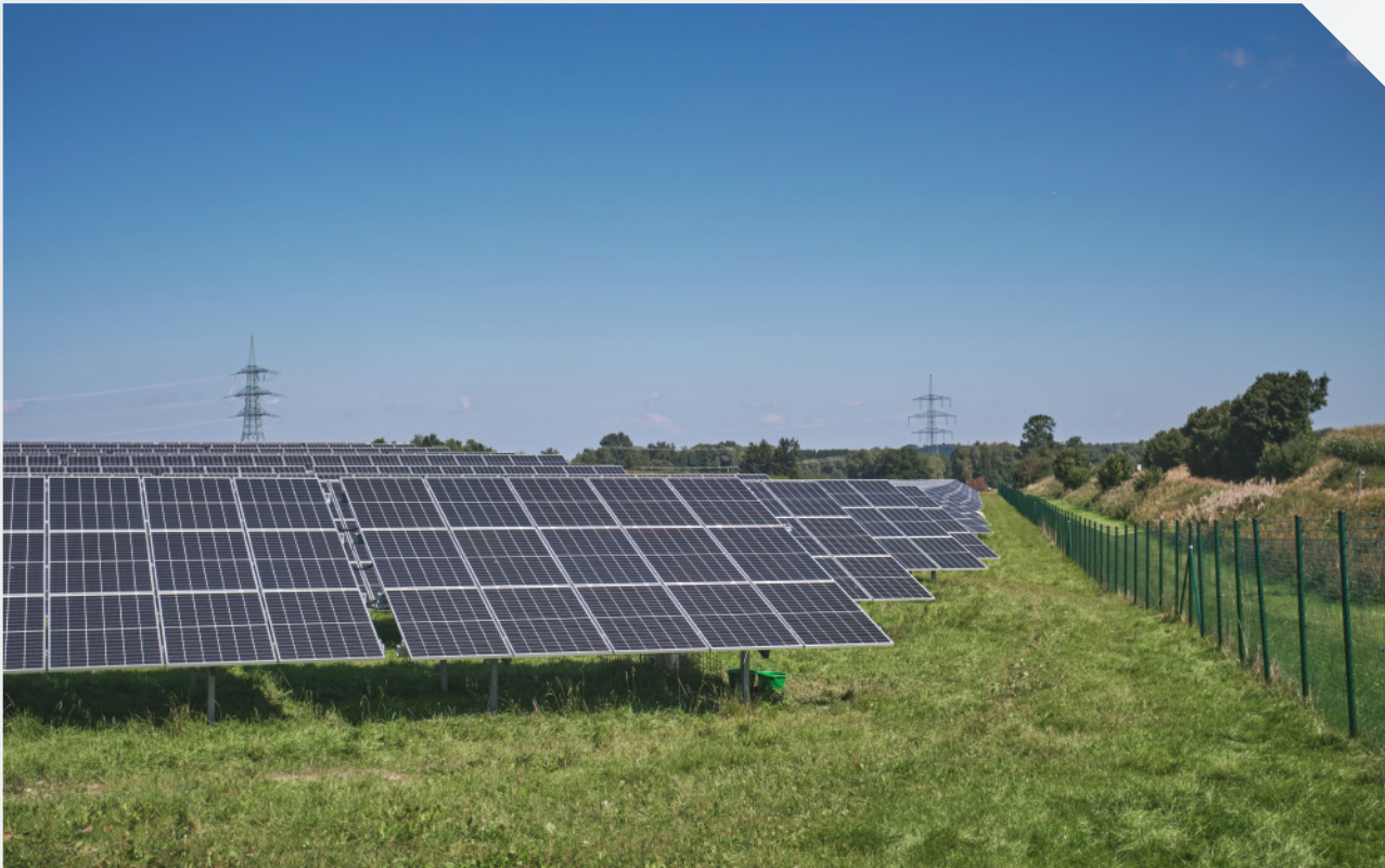
300MW+ 📍 Project Location: Kyushu, Japan 📋 Module Type: Solar N Plus N-Type 435W 📅 On-grid Date: 2024.1-2024.12
